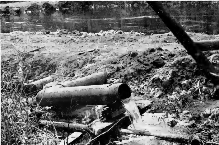
Oil field brine being discharged to fresh water bodies. By orders of the Louisiana Department of Conservation and by the Louisiana Stream Control Commission in 1968, discharge of oil field brines to fresh water bodies is no longer allowed.
